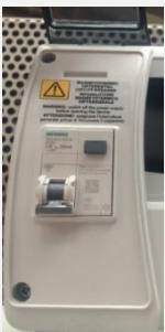
Picture 1 - Differential circuit breaker for the protection and disconnection of the refrigeration unit
