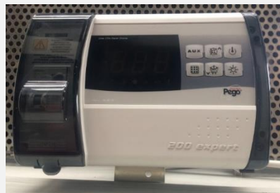
Picture 2 - Control panel of the refrigeration unit
